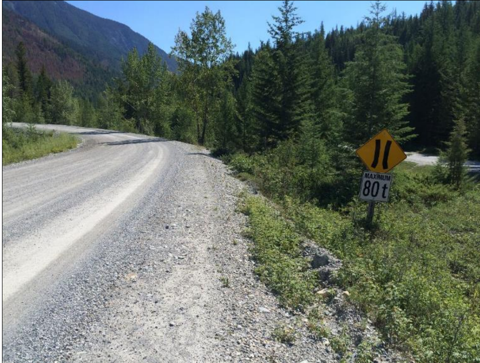
Photo #31 Load posting sign ahead of Abutment 1
